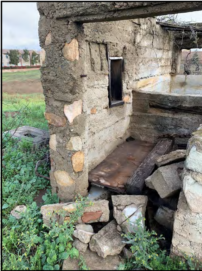
The pump house was divided into two parts: the back half was the water cistern and the front half was the cold storage. The cement roof has collapsed and the door was removed.
